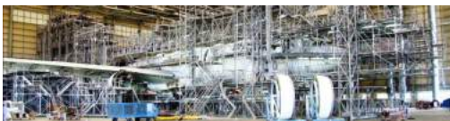
Docking system for Thai Airways, U-Tapao Airport
